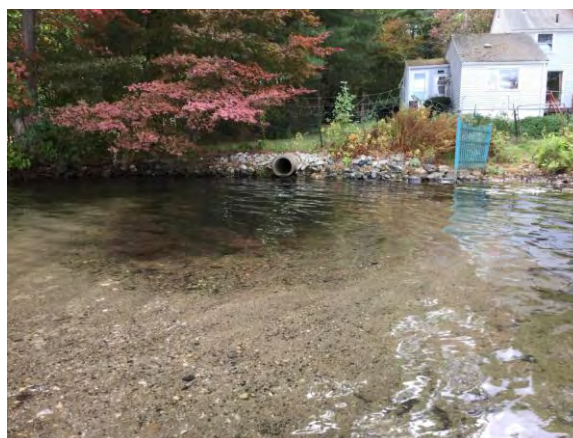
Outfall and sediment deposit in pond.
