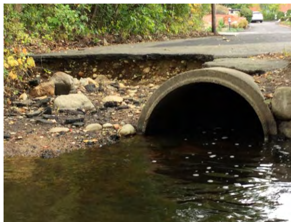
48" concrete culvert conveying flows of Jennings Brook. Note erosion next to culvert.
