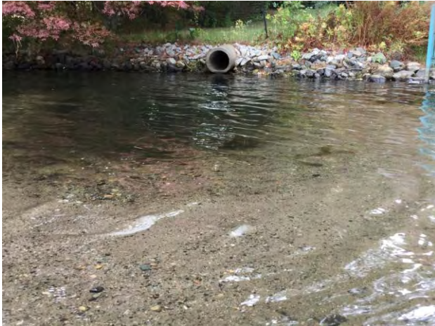
Outfall and sediment deposit in pond.
