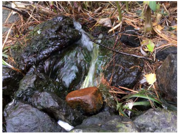
Water bubbling from shoreline near outfall, which is dry.
