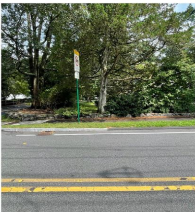
Asphalt to granite curb, Kenilworth
