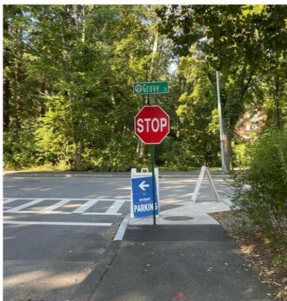
Asphalt to granite curb, no grass strip
