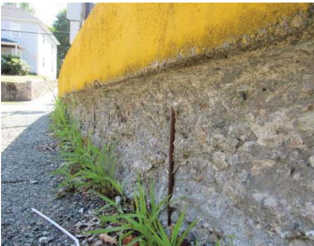
Image 61 – East retaining wall exposed rebar
