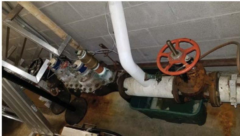
Water Meter Serving the Building
