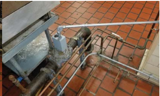
Hood Gas Shut-Down Valve
