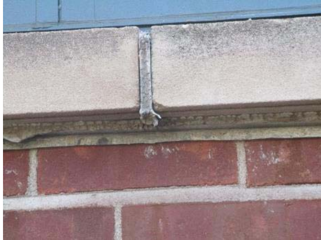
Image 15 – Sealant between limestone and flashing
