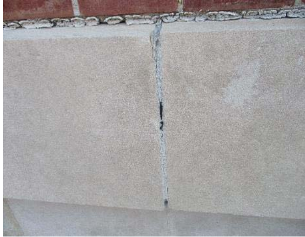
Image 49 – Deteriorated sealant joints
