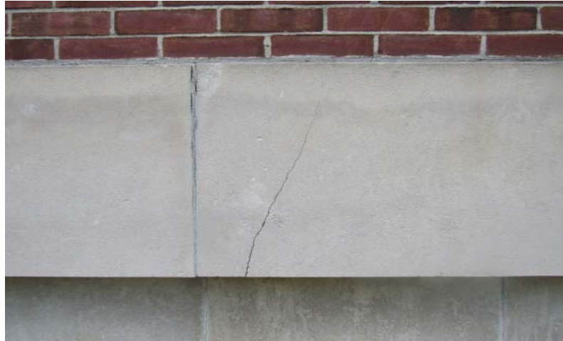
Image 42 – Crack in limestone band course
