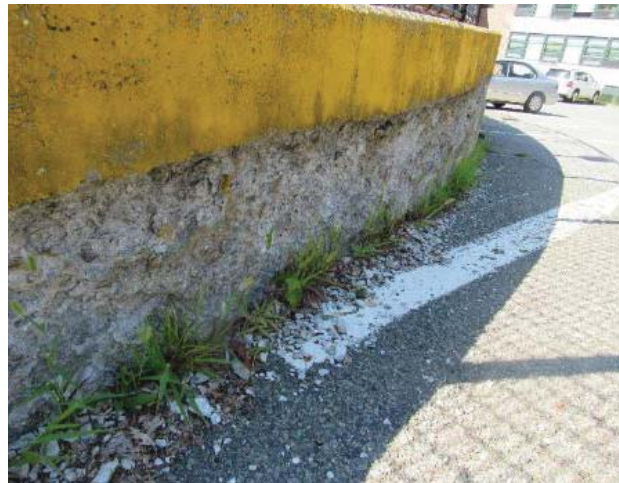
Image 60 – East retaining wall concrete spall
