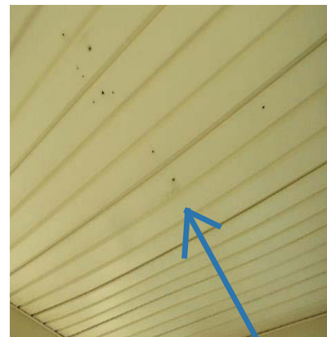
Image 77 – Water dripping from soffit (arrows)
