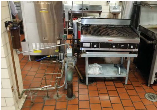
Exposed Gas and Water Supply Piping
