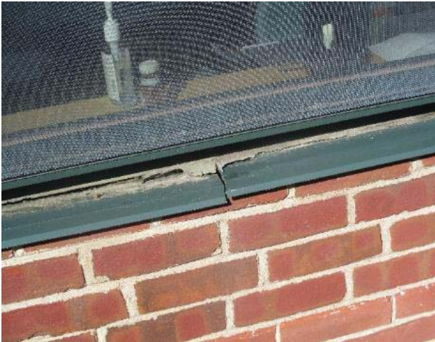
Image 57 – Deformed window sill flashing
