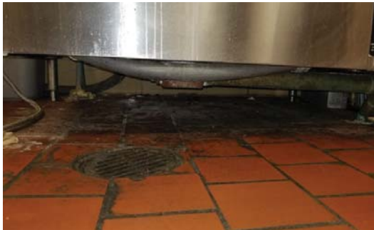
Floor Drain and Dishwasher Drain
