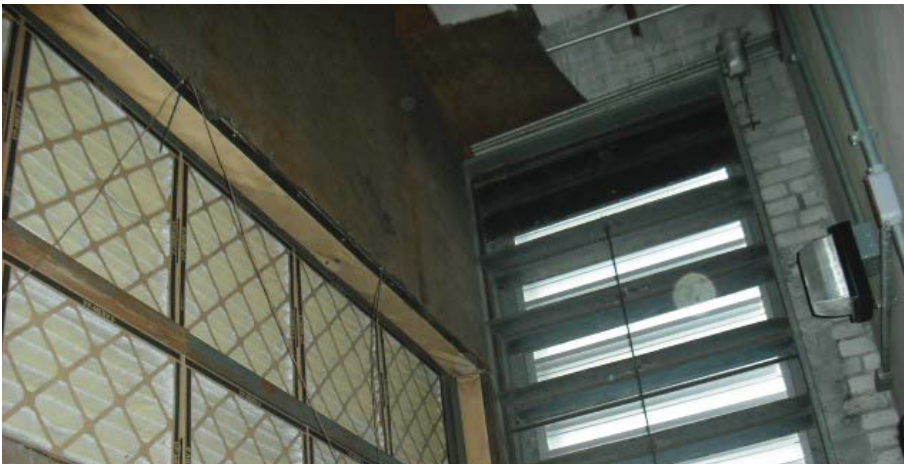
Image 8 – Auditorium air handler with duct-mounted filters
