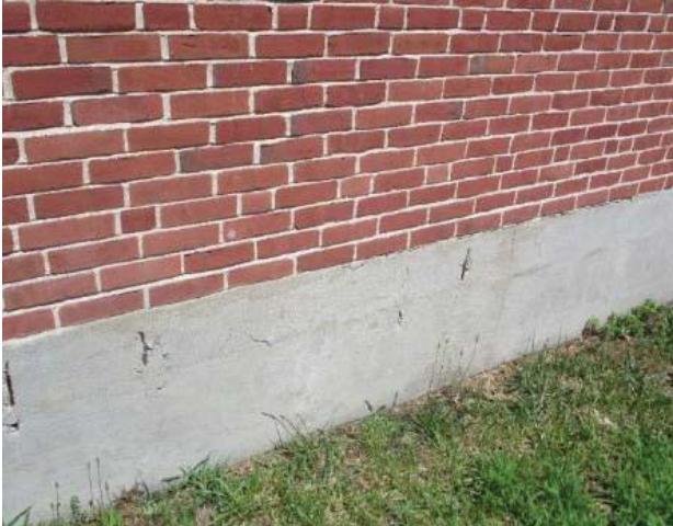
Image 24 – Exposed reinforcing steel
