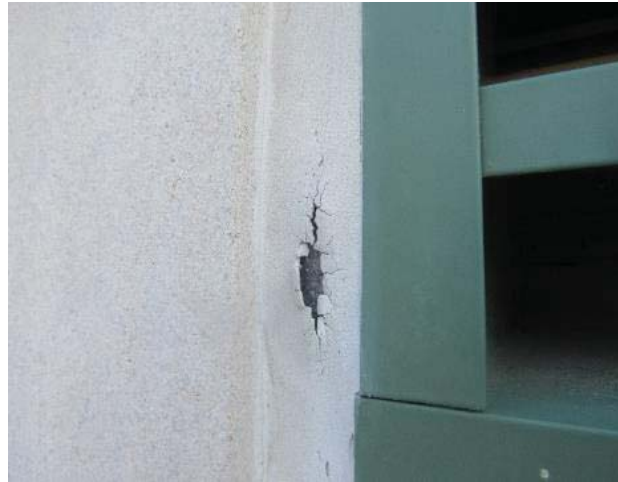
Image 58 – 1966 addition failed sealant joints
