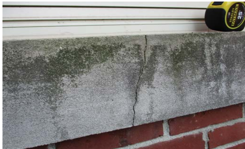
Image 43 – Crack in limestone sill
