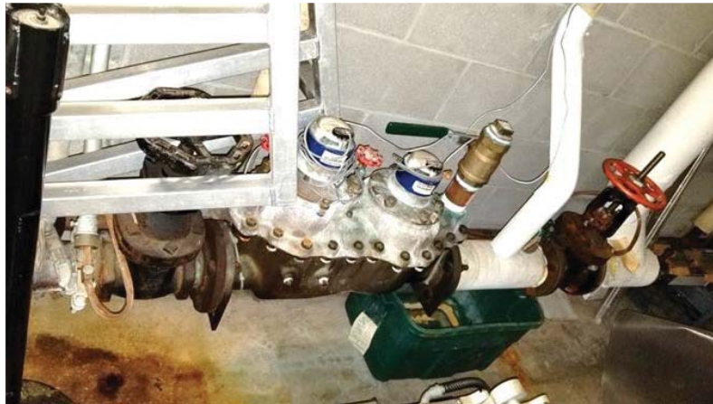
Water Meter Serving the Building
