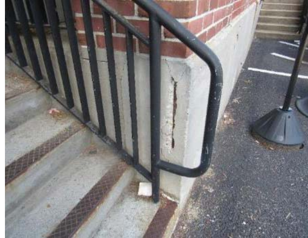
Image 25 – Exposed reinforcing steel
