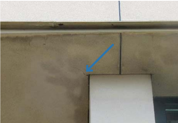
Image 65 – Cracks through the stucco soffit
