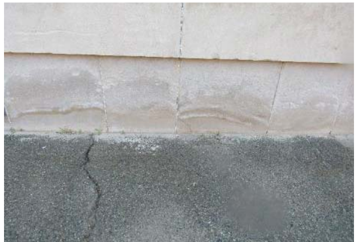
Image 68 – Spalled limestone panels, cracked bituminous asphalt pavement, and deteriorated limestone panel sealant joints
