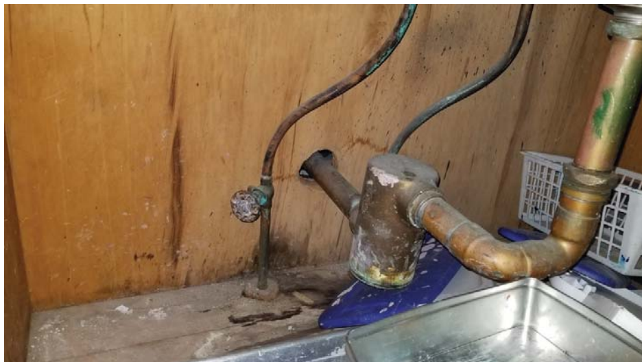
Piping Below Sink in Art Room 304B
