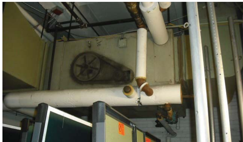
Image 1 - Air handler in east mechanical room - Gym A
