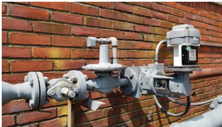
3 Million BTUH Natural Gas Pressure Regulator and Meter
