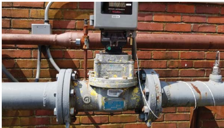
18 Million BTUH Boiler Plant Natural Gas Meter
