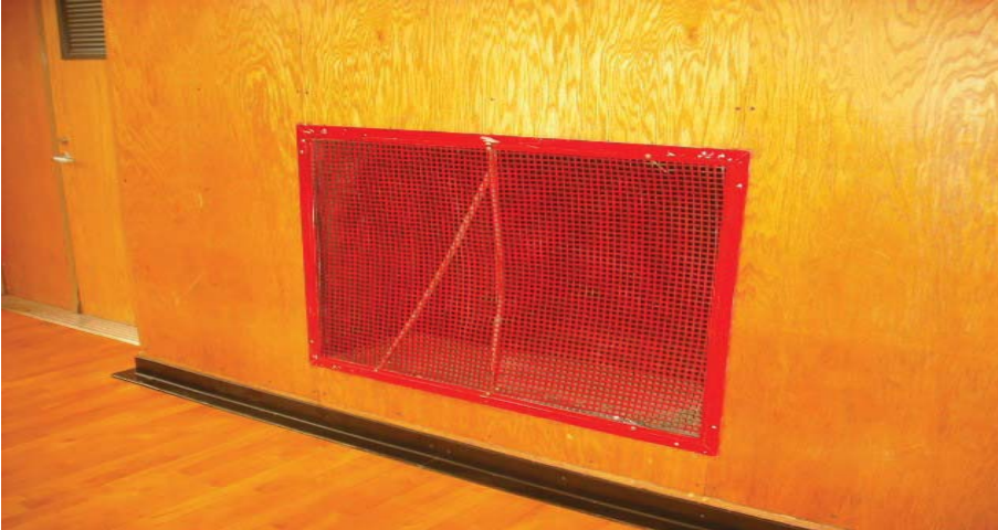
Image 3 – Damaged return grille - west side Gym A
