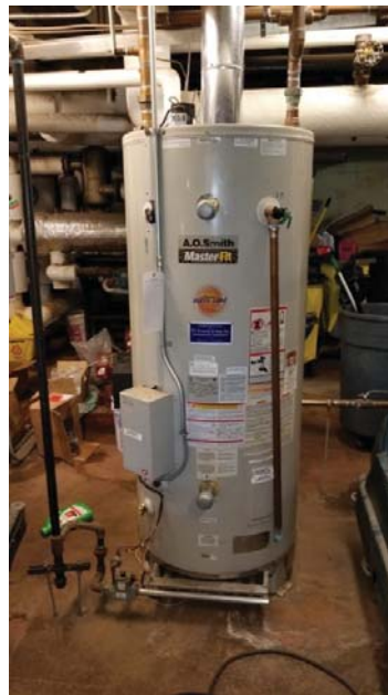
Gas Fired Water Heater
