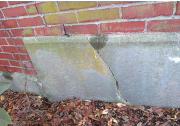
Image 63 – Same crack shown in Image 62 at foundation
