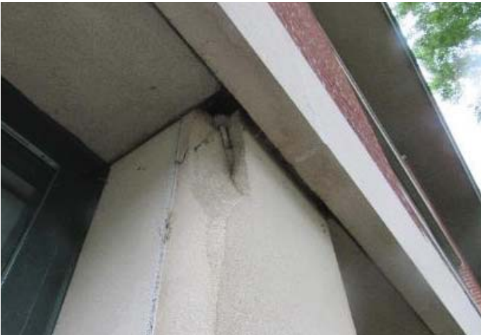
Image 38 – Full panel depth spall
