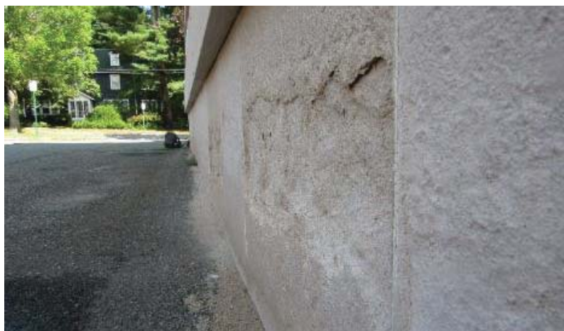
Image 35 – Limestone erosion at grade near parking area at the 1966 Addition
