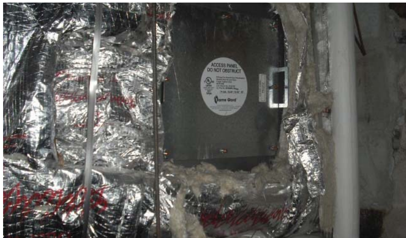
Image 11 – Kitchen cooking hood exhaust duct in auditorium mechanical room
