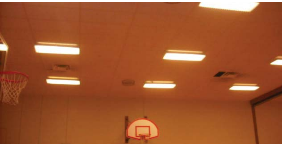
Image 5 – Ceiling diffusers in Gym B
