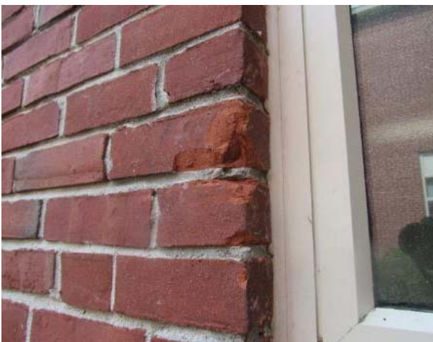
Image 28 – Small shallow area and spall does not penetrate into the mid-depth of the brick
