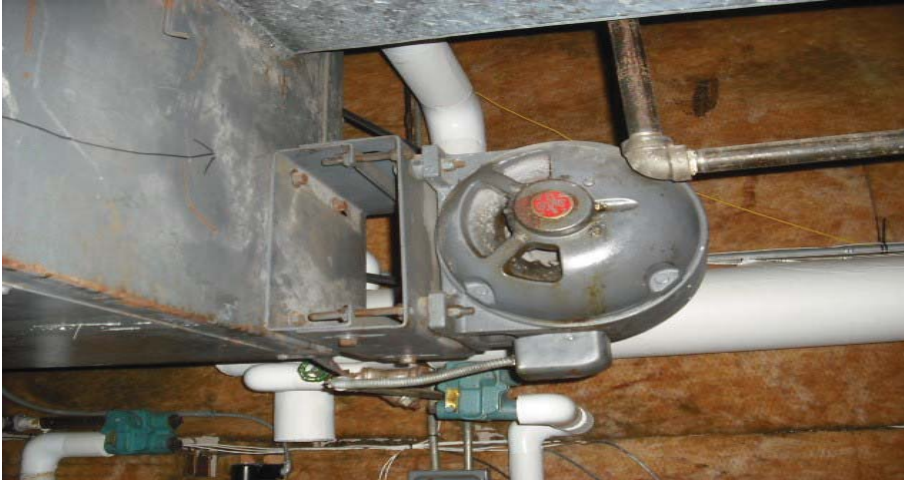
Image 7 – Auditorium air handler
