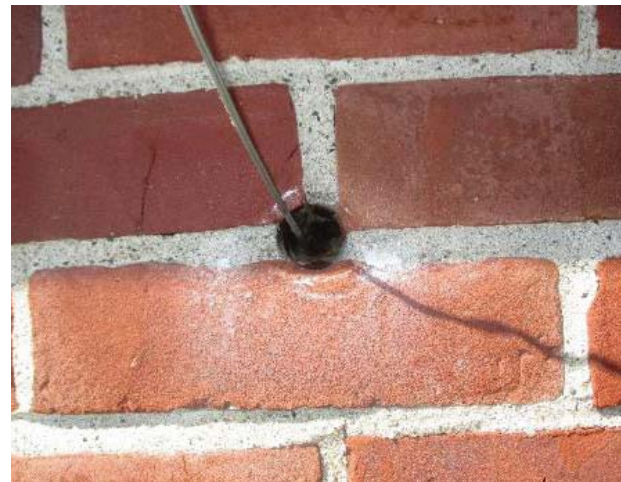
Image 53 – Empty holes in the brick masonry
