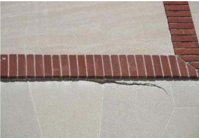
Image 40 – Large spall at south entrance
