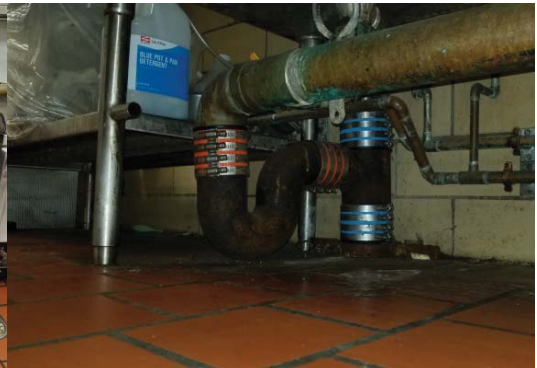
Drainage Piping Below 3-Bay Sink
