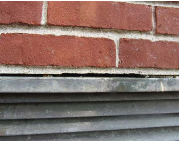
Image 50 – Gap between the mortar and vent frame
