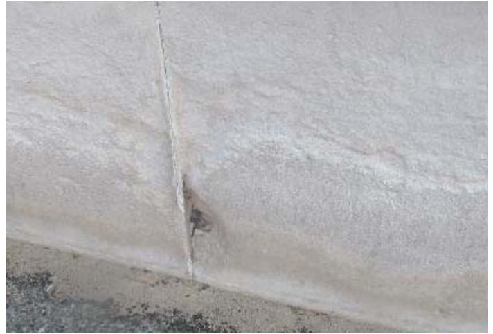
Image 37 – Exposed anchor at spall
