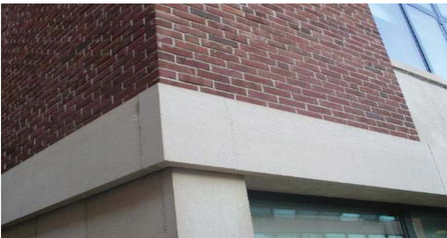
Image 47 – Location two: Limestone crack
