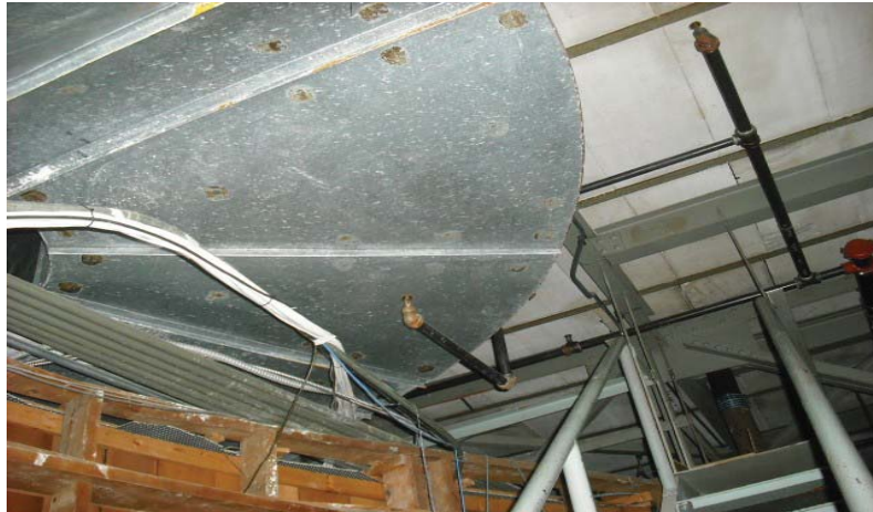
Image 10 – Uninsulated auditorium supply ductwork
