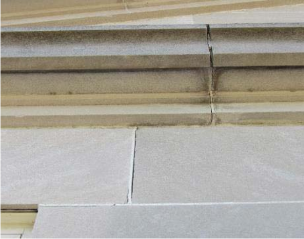
Image 48 – Deteriorated limestone mortar joints
