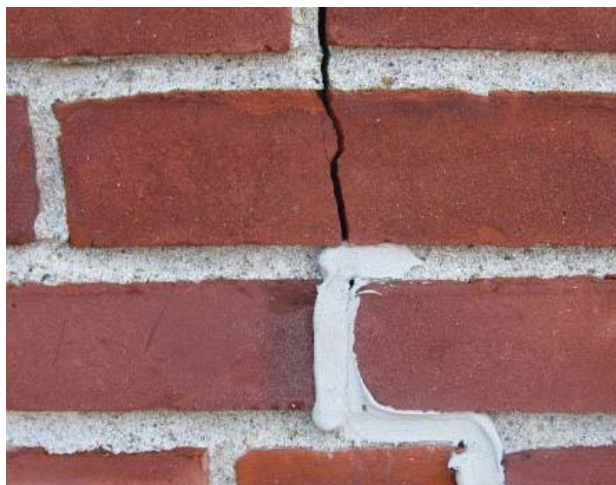
Image 29 – Crack that is approximately 6 ft long with the lower 3 ft covered with sealant, same location as Image 30
