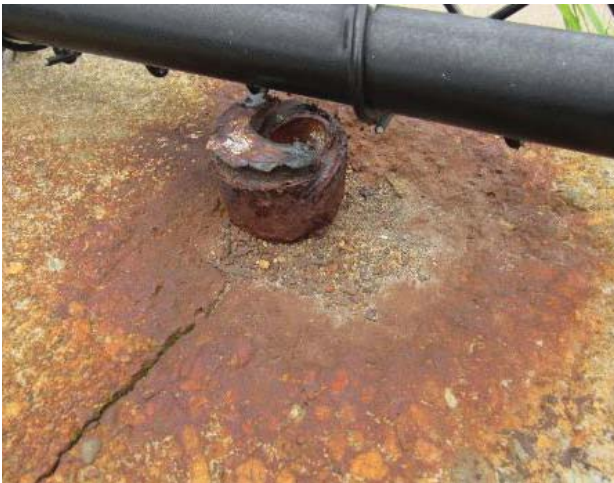
Image 59 – Abandoned existing fence posts embedded in the retaining wall
