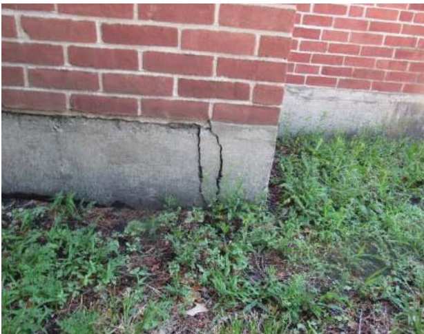
Image 26 – 1/4 in. wide cracks
