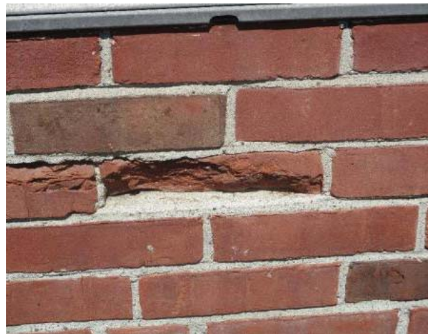
Image 27 – Spalls that extend into the mid-depth of the brick
