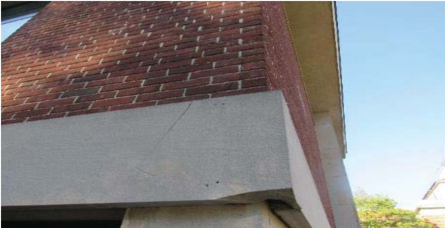
Image 45 – Location one: Limestone crack
