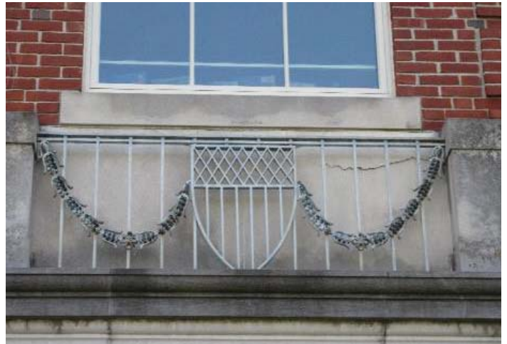
Image 39 – Large spall at north entrance
