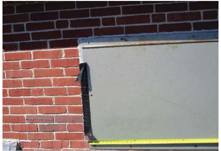
Image 64 – Temporarily weatherproofed with tape
