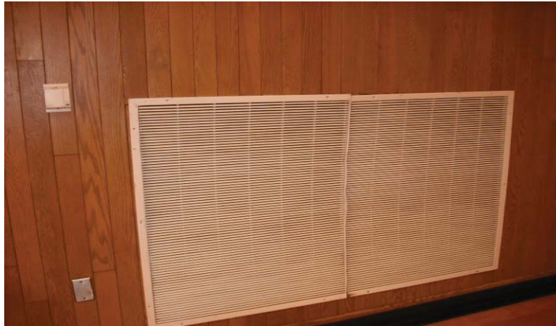
Image 4 – West air handler for Gym B
