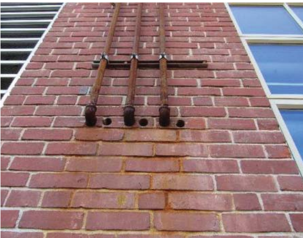
Image 52 – Empty holes in the brick masonry
