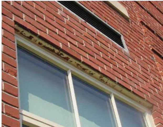
Image 51 – Some surface rust where the coating has failed
