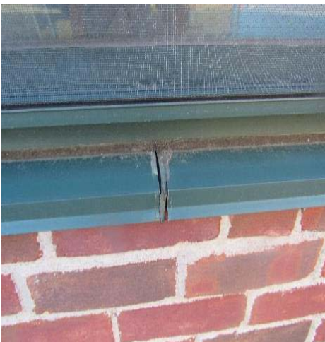
Image 56 – 1958 Addition failed sealant joints
