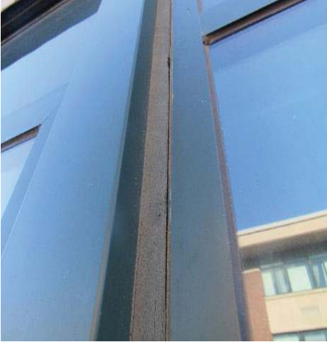
Image 54 – 1958 Addition failed sealant joints
