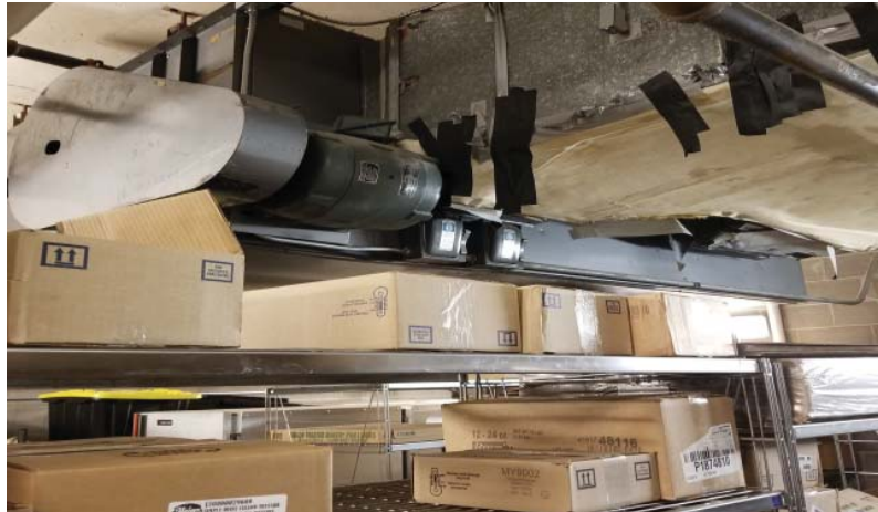
Image 10 – Make-up air handler
