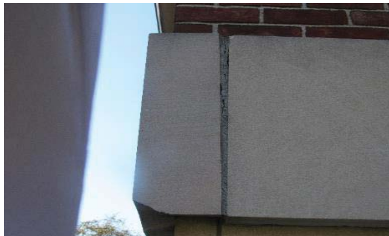
Image 44 – Location one: Limestone crack
