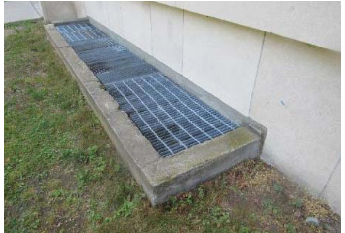
Image 66 – Cracked or missing the 2 in. bluestone caps
