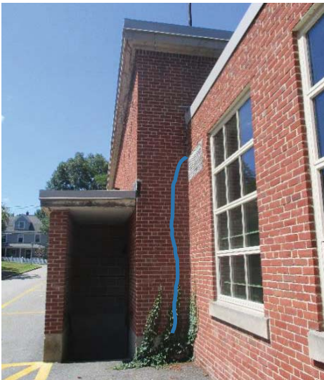
Image 31 – Crack that extends from the foundation to the edge of the roof on the 1958 Addition (represented by blue line)
