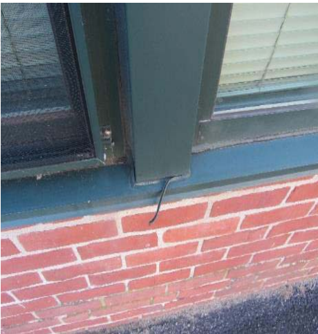
Image 55 – 1958 Addition failed sealant joints
