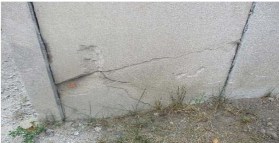
Image 46 – Location one: Limestone crack
