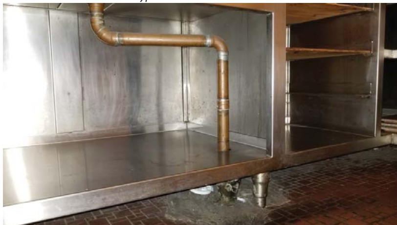
Floor Drain with Funnel below prep sink
