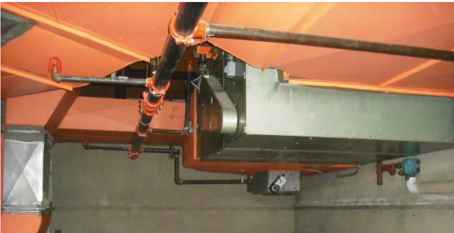
Image 4 – West air handler for Gym B
