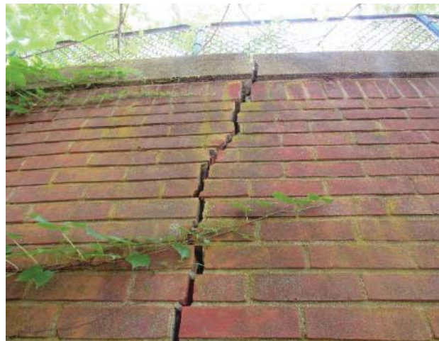
Image 62 – One crack was 1-1/2 in. wide
