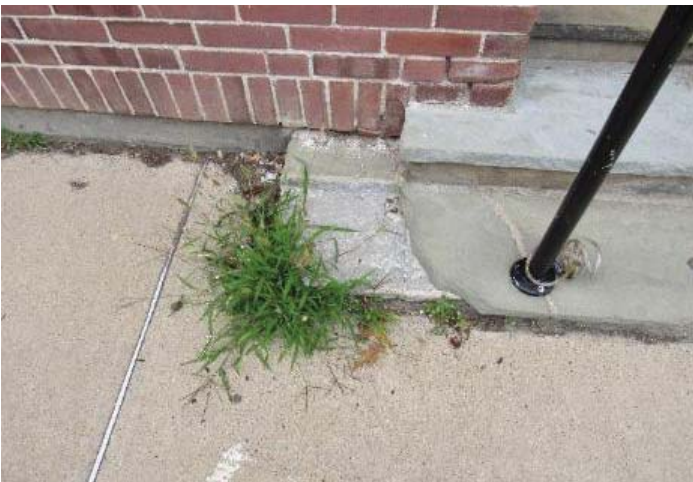
Image 67 – Cracked bluestone at stairs
