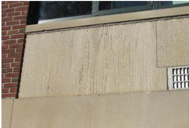
Image 34 – Some panels are weathered.
