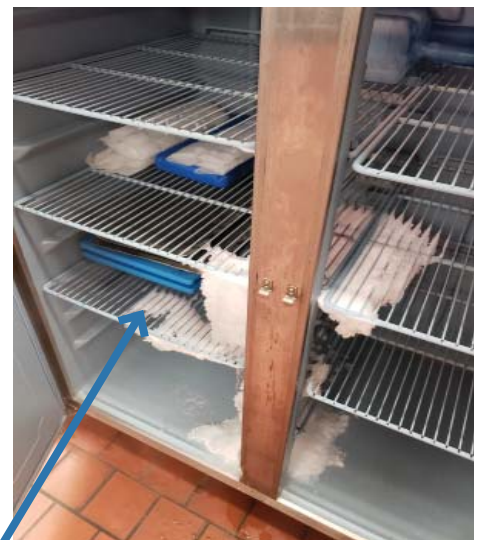
Image 9 -Reach in Freezer
