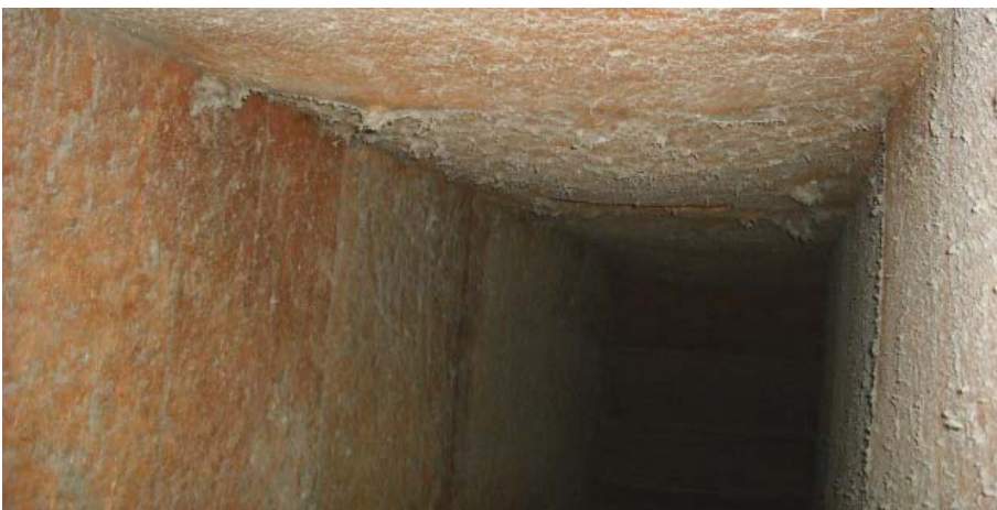
Image 9 – Dirty auditorium ductwork
