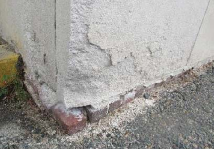
Image 36 – Limestone erosion at grade near parking area at the 1966 Addition
