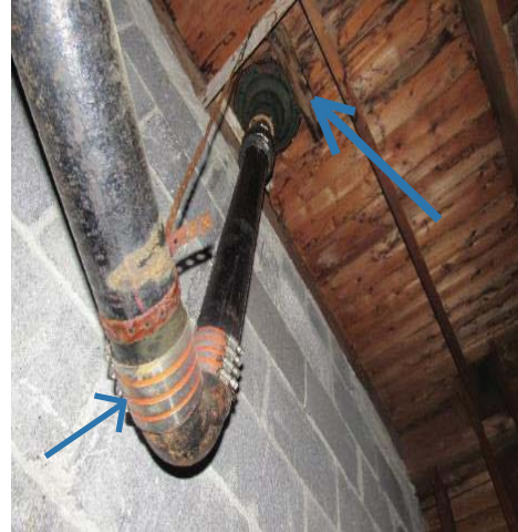
Image 75 – Water dripping from drain (arrows)
